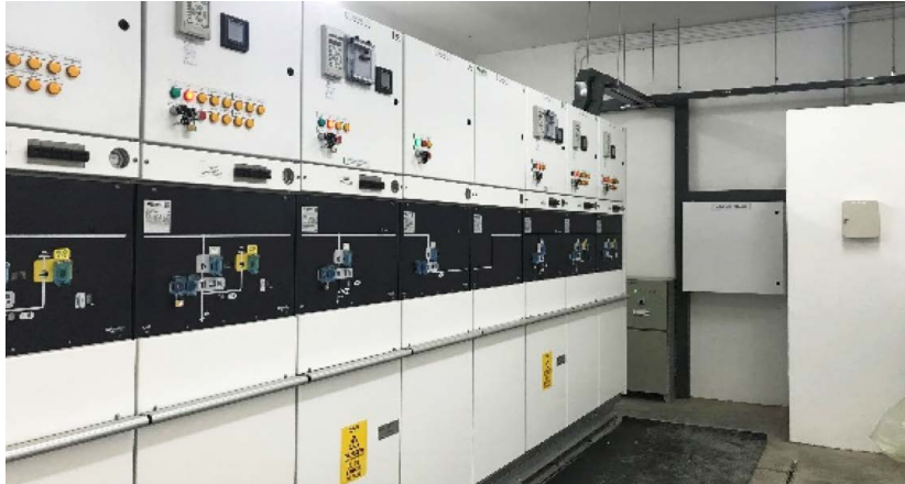
Orchard Rendezvous Hotel, High Tension Switchgear
