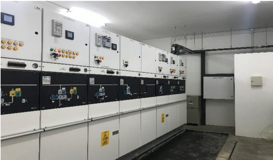
22KV High Tension Switchgear
