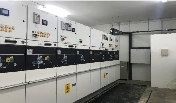
22KV High Tension Switchgear
