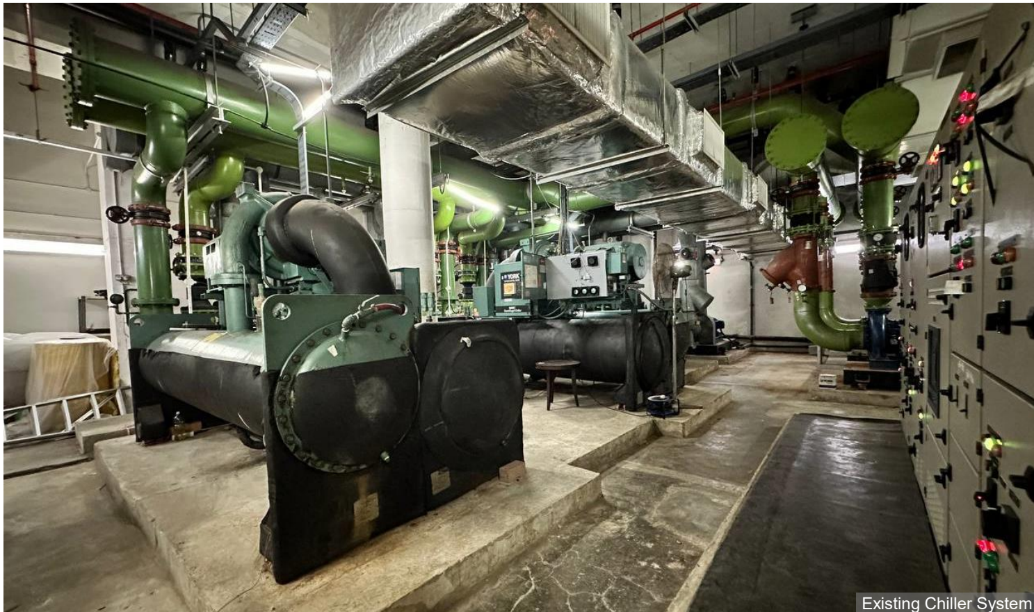
Existing Chiller System
